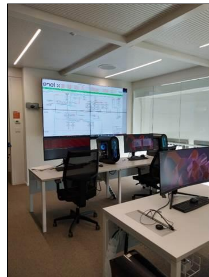
3- XLAB Control Room
