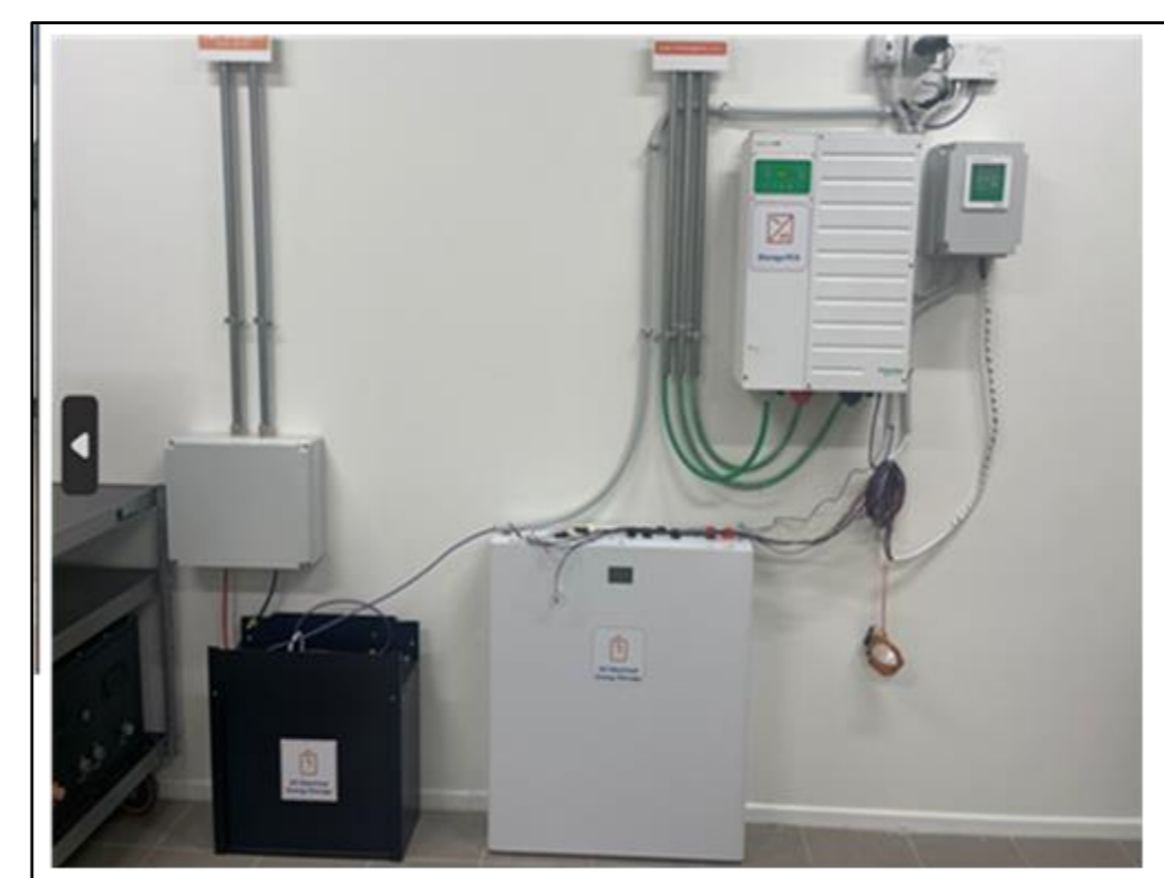
6- RES Battery- Pylontech- IEEE2030.5XWPRO Gateway
