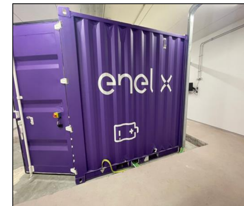
4- Utility scale Battery-SOCOMEK
